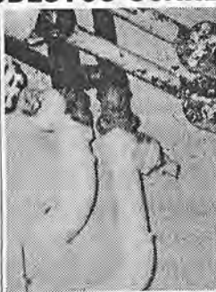
from heating pipes had been ripped out by council contractors (TO 867).
